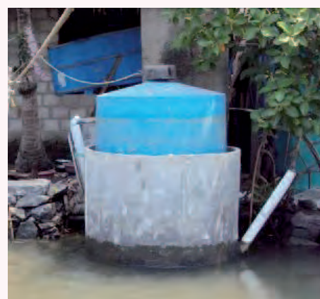
Figure 5: Biogas plant discharging directly into the backwaters
