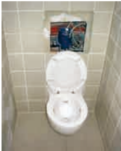
Figure 5: Ceramic vacuum toilet with built-in vacuum valve at Burg Lenzen
