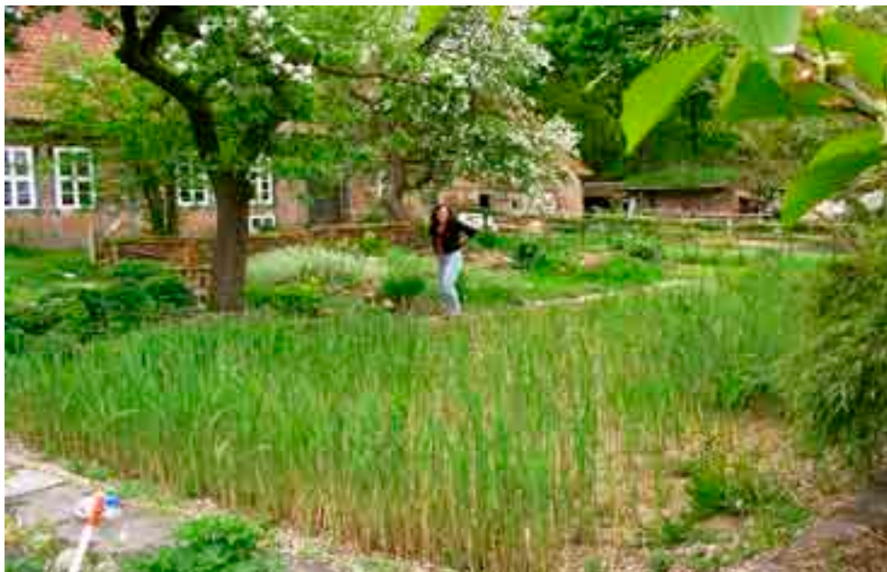
Figure 3: Garden-integrated vertical-flow reed bed for all-season greywater purification (10 pe) (Neumühlen/Böhme, Lower Saxony; Photo: B. Ebeling)
