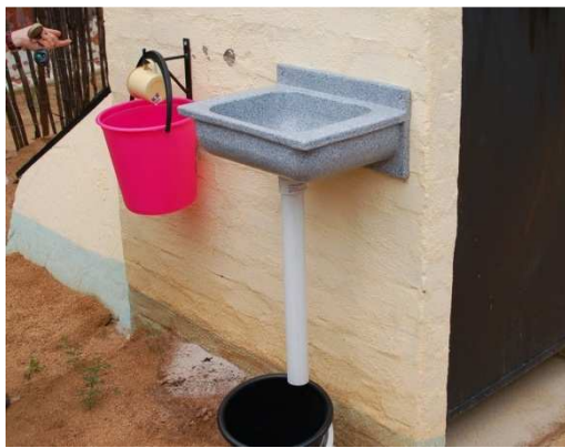
Fig. 6: Basic handwashing facilities attached to the toilets. The pink bucket provides fresh water, the cup is used to fill the basin and the black bucket collects the greywater which can be used for irrigation (source: GIZ, Kleemann, 2011).
