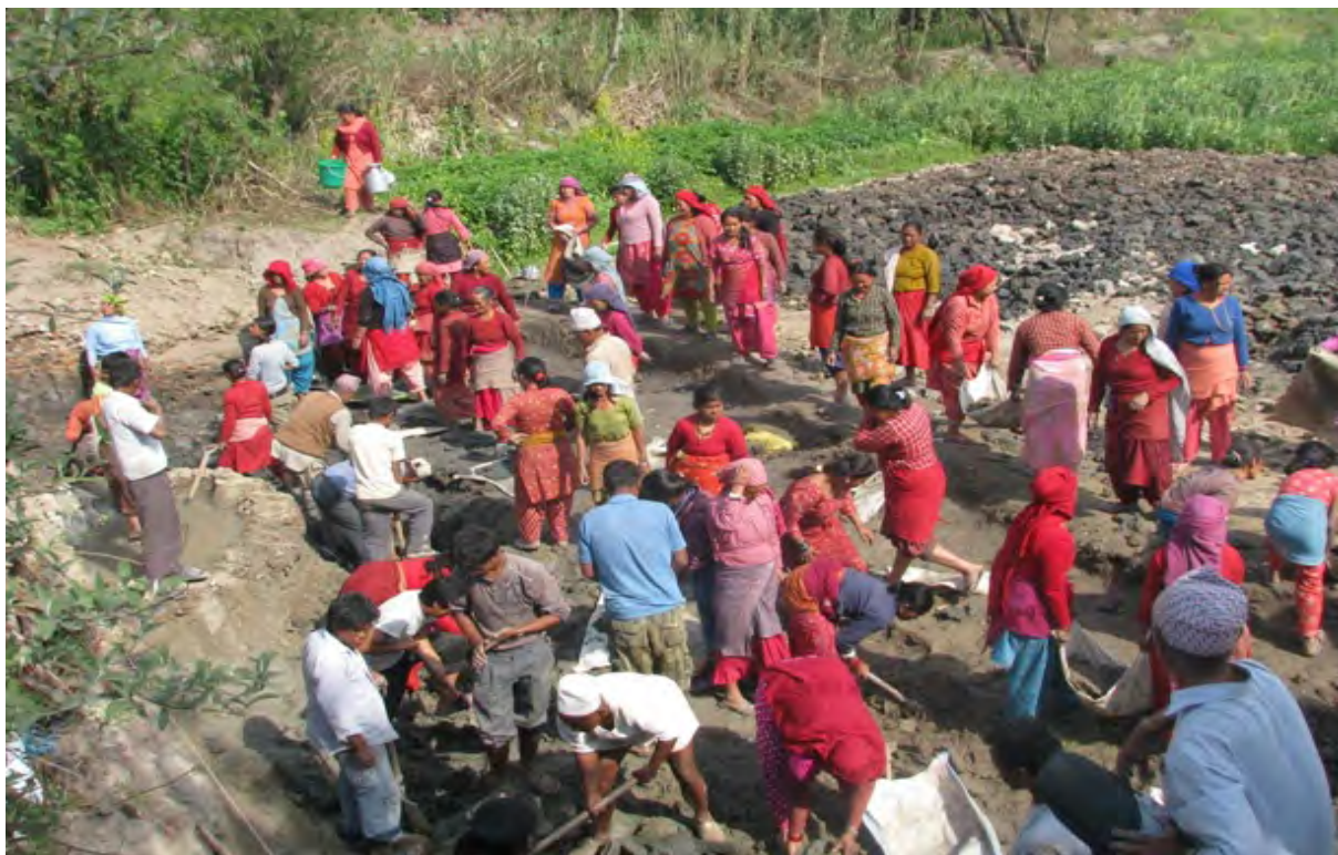
Figure 9: Community self-help efforts - preparing the ground for the decentralised treatment plant (constructed wetland), Nala (Nepal) (Source: M. Sherpa).
