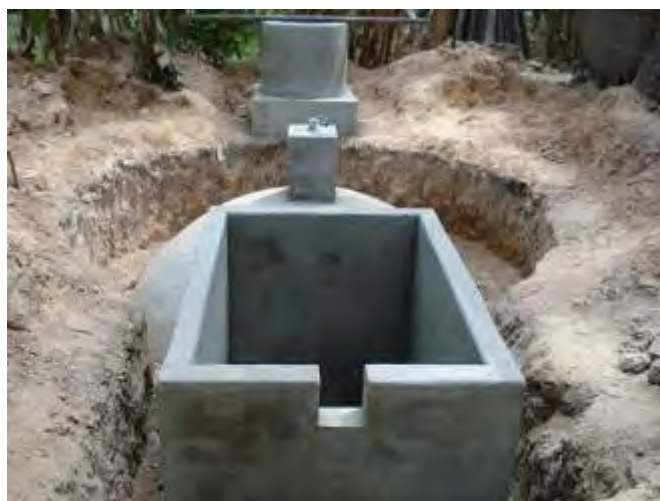
Figure 4. A nearly completed biodigester, showing the mixing tank (rear), digester (middle), and outlet (front)
