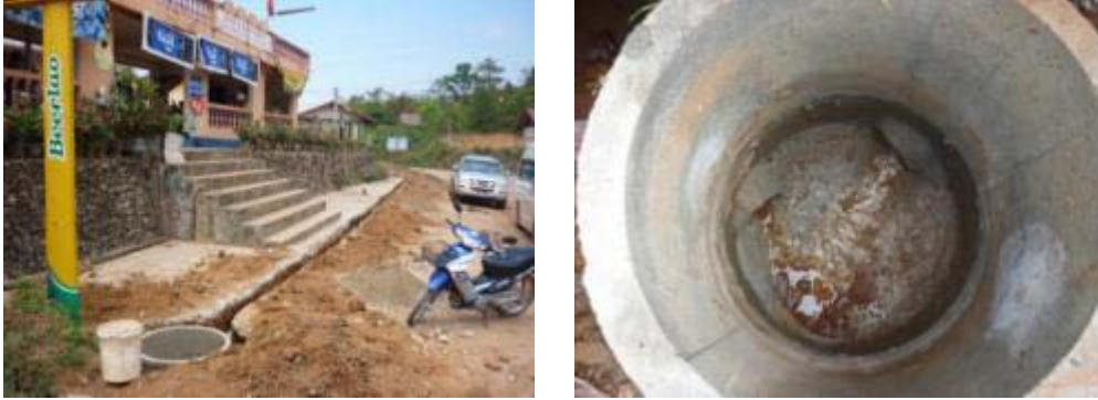
Figure 5. Photo of the construction of the simplified sewer (left) and a manhole along its path (right)
