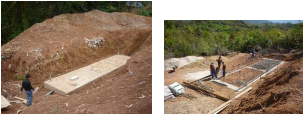
Figure 6. Photo of the completed WTP (left) and the sludge drying beds under construction (right)
