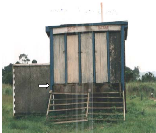
Figure 2: The old disused VIP toilet (note the raised structure due to ground water table)
