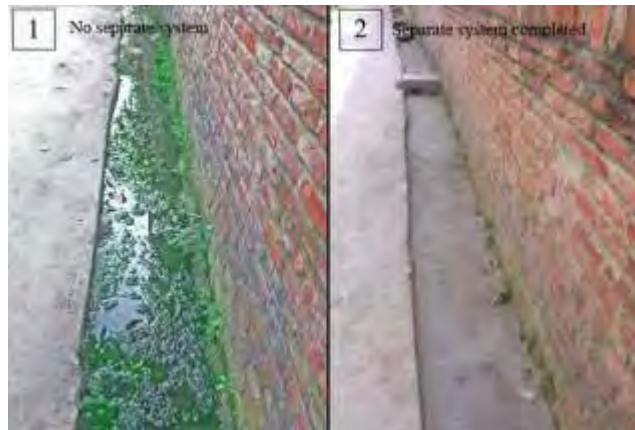
Figure 4. A drainage canal before and after the installation of the DEWATS & gravity-fed sewer
