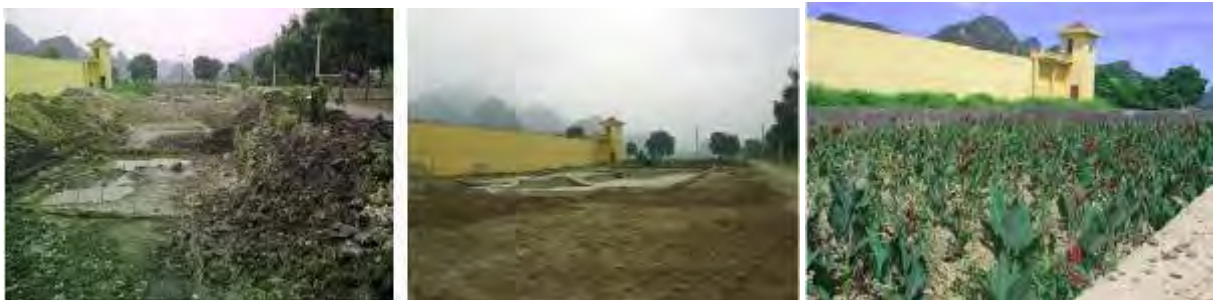
Figure 4. Photos of the Ninh Khanh Prison project under construction, as well as the completed HGF
