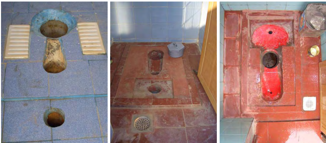
figure 16: “3-hole system” at ACTS eco-friendly demonstration toilet in Rajendra Nagar, Bangalore (left), “3-hole system” at Navsarjan Primary School in Dhandhuka taluka (center) and prefabricated squatting pan that allows source-separate collection of urine, feces and anal cleansing water (design supported by UNICEF) (right)
