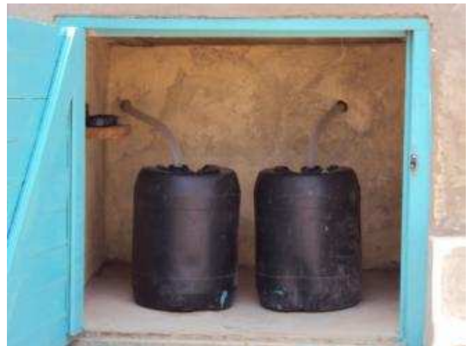
Fig. 11 Two 20 L urine containers with flexible hoses in a vault attached to the UDDT at Mwala Primary School, Ukambani (source: Johannes Orodi, GTZ Kenya, Oct. 2009).
