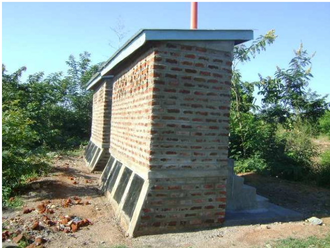
Fig. 10 Rear view of 2 toilet blocks with inclined vault doors and ventilation opening which also provide additional light inside the cubicle (source: Paul Mboya, GTZ Kenya, Jan 2009)
