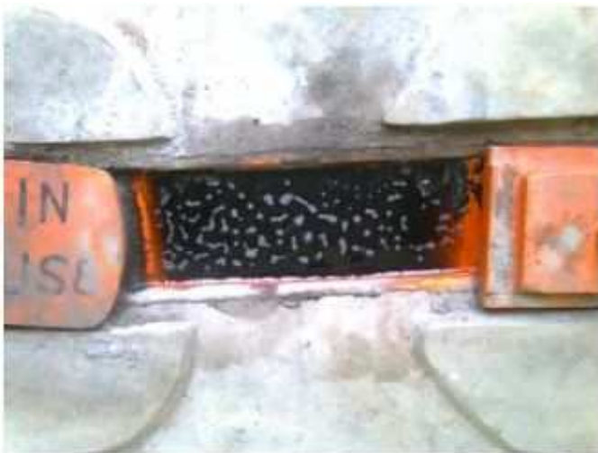
Fig. 14 A urine pipe of a urine diversion squatting pans got blocked with ash at Muslim Primary School, Mumias. Faeces drop holes are covered with lids on the left and right in this photo (source: Laura Kraft, GTZ, June 2010).
