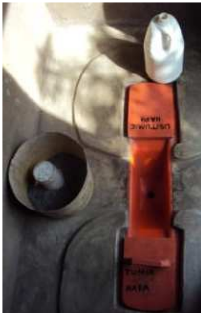
Fig. 7 Plastic urine diversion squatting pan with concrete footsteps inside a UDDT. Urine is collected in the centre; the two lids are covering the two faeces vaults (source: Laura Kraft, GTZ, June 2010).
