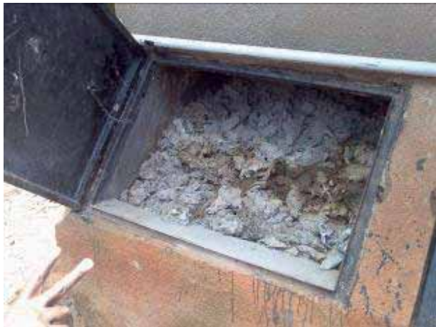
Figure 1: Dried faecal material contaminated by water through the rear trap door.
