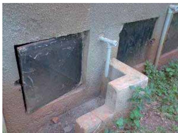
Figure 4 The vertical trap door, with reduced heating from the sun.
