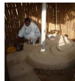
The double vault UDDT in local material except slab and vent pipe.
