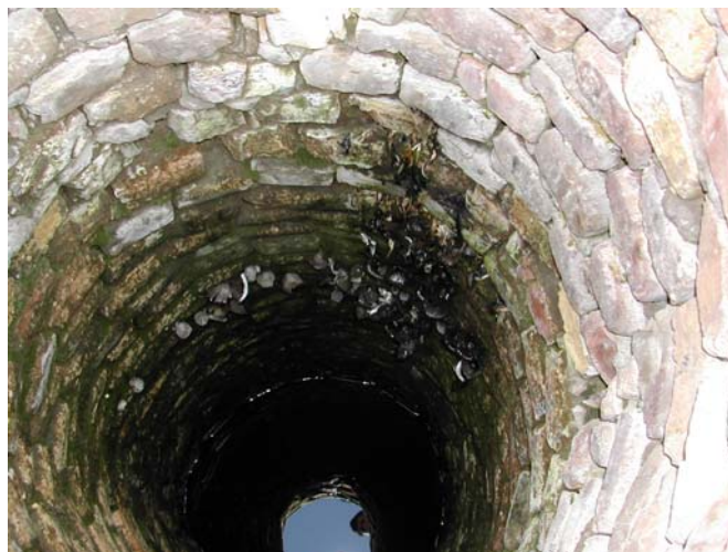
Figure 3.8 Mushrooms on brick wall of the above dug well contaminating the drinking water
