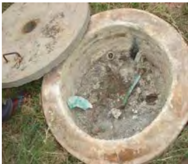
The leakage at the outlet pipe at the Ecole Secondaire Ste Bernadette de Kamonyi
