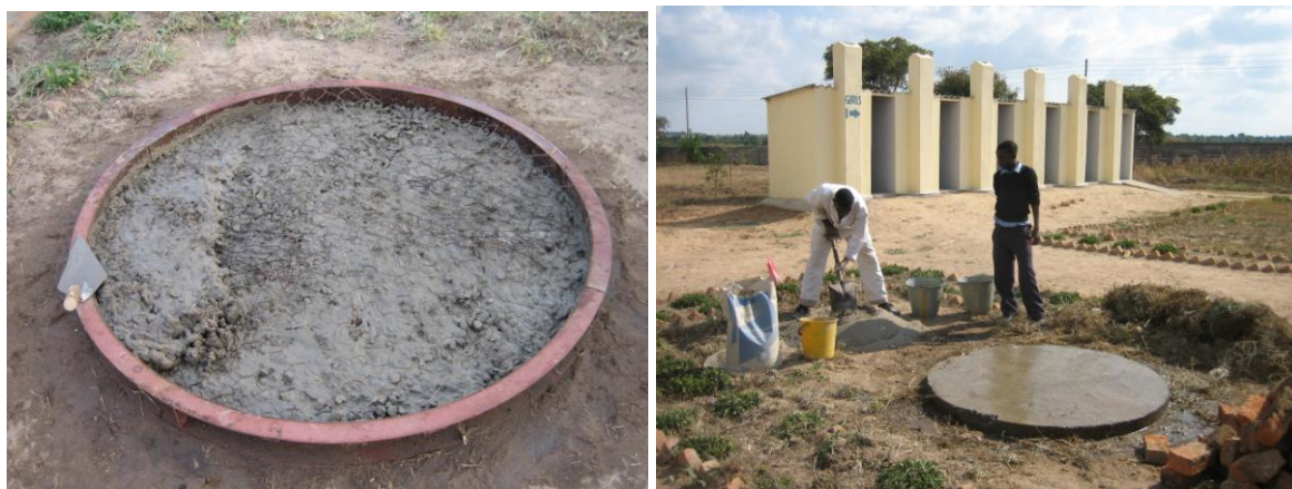
The strong base slab (diameter 1.4m) is cast in a suitable position
