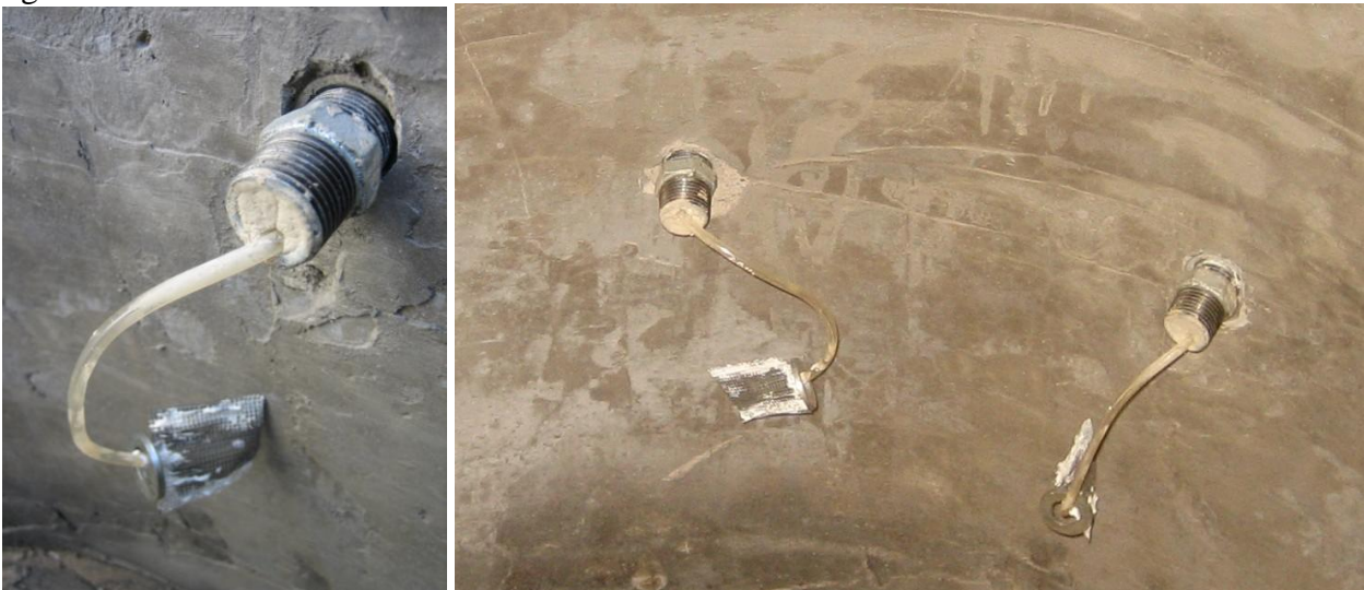
The water restricting units inside the tank
