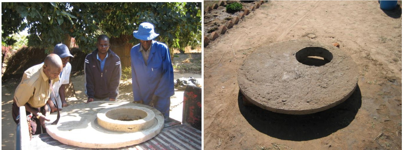
After curing the cover slab is lifted and moved to the tank site. The underside is washed down.
