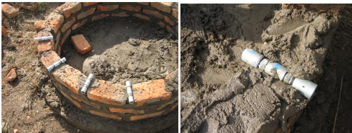
The steel pipes are laid through the brick all above the third course of bricks. A strong cement mortar is used to bond the bricks around the steel pipe. The pipes are placed on one side of the tank. A water catchment area is built beneath the taps which lead to a water run-off. The steel pipe should protrude slightly from each side of the brick wall.
