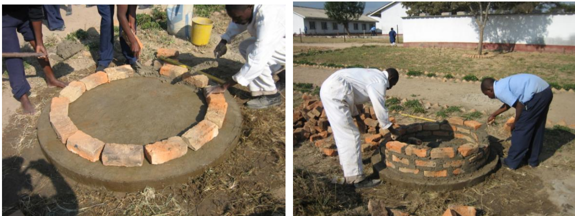
The first three courses of bricks are laid down with an external diameter of 1,2m in strong cement mortar.
