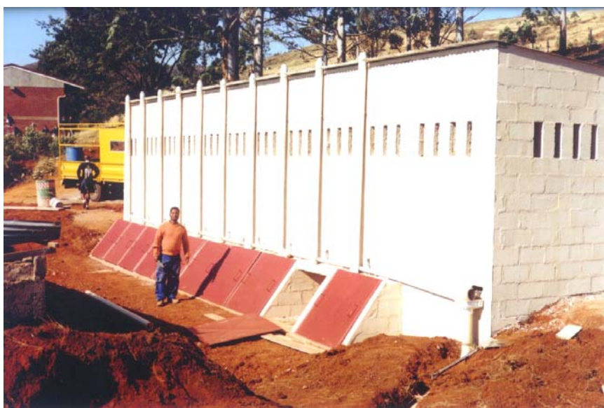
Figure 6: Construction details: left, handwashing trough and part of urinal; right, urine tank; below, nearly completed structure showing vaults
