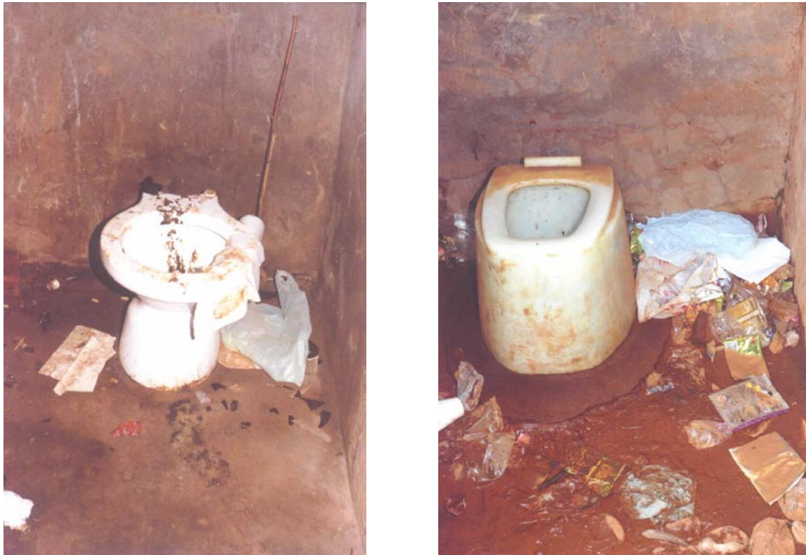
Figure 1: The existing school latrines
