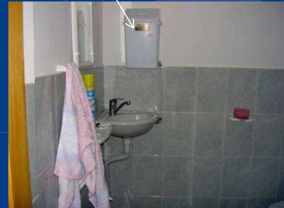
Hand wash basin in Moldova with water reservoir
