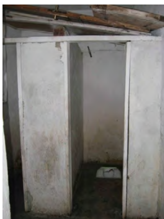
Figure C.19: school toilet boys with broken door (Niebel 2011)
