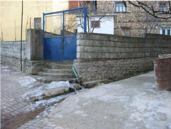
Figure C.40: Rain water channel in village Lin (Niebel 2012)
