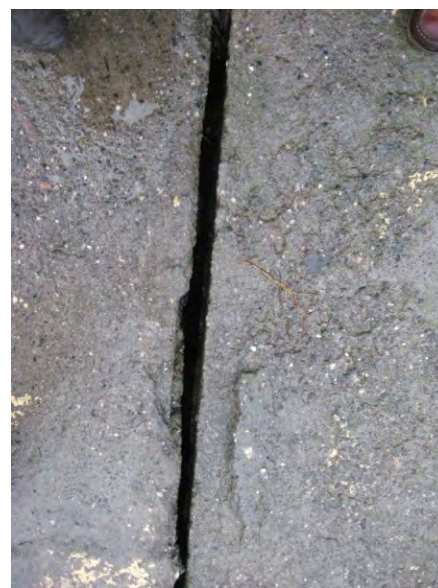
Figure C.22: space between concrete cover of the septic tank allows rainwater to flow into the tank (Niebel 2011)
