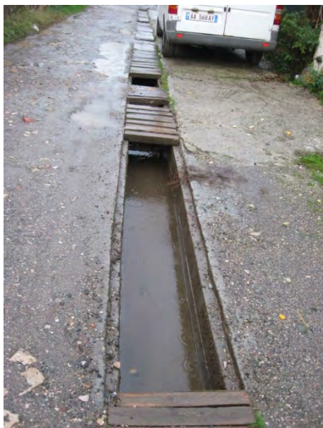
Figure C.12: Rain water channel of Ishull Shëngjin is only partly covered with wooden plates (Niebel 2011)
