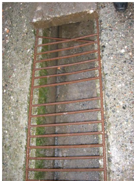
Figure C.13: Rain water channel in the village Ishull Shëngjin (Niebel 2011)
