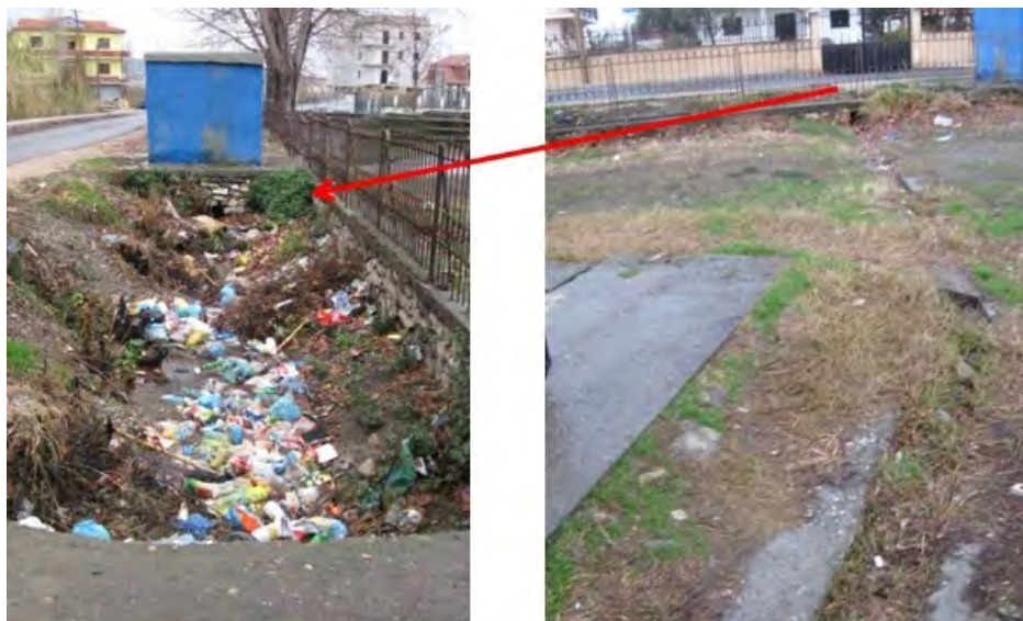
Figure C.17: Rain water trench at the school yard and the rainwater channel next to the yard, both blocked with waste (Niebel 2011)
