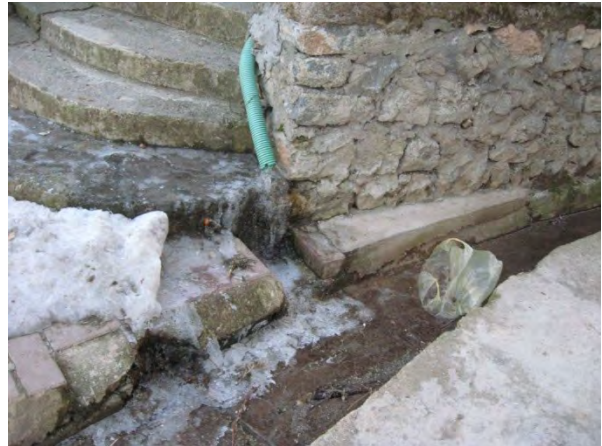
Figure C.41: Private water discharge into rain water channel (Niebel 2012)
