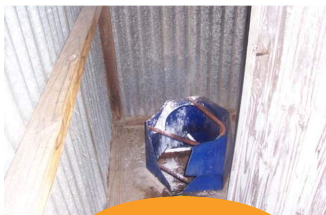
Toilet with broken pedestal
