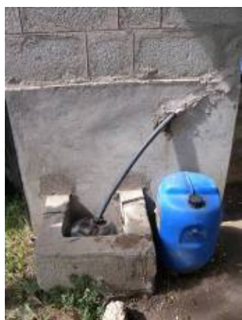
Figure 20: Urine storage in closed storage tank (Arusha, Tanzania).
