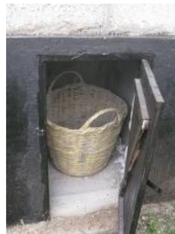
Figure 19: Container for storage of faeces (Arusha, Tanzania).
