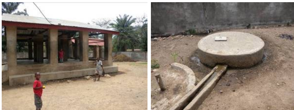
Figure 6: The slaughter house and the unsealed tank for wastewater.
