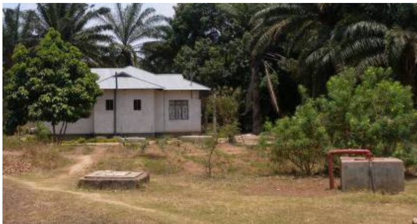
Figure 3 Borehole at police station in close vicinity to an unsealed septic tank.
