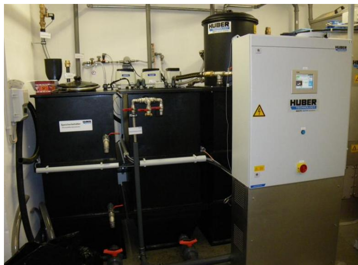
Figure 8: Greywater treatment plant in the GIZ's main building in Eschborn/Germany; (picture by K. Löw)
