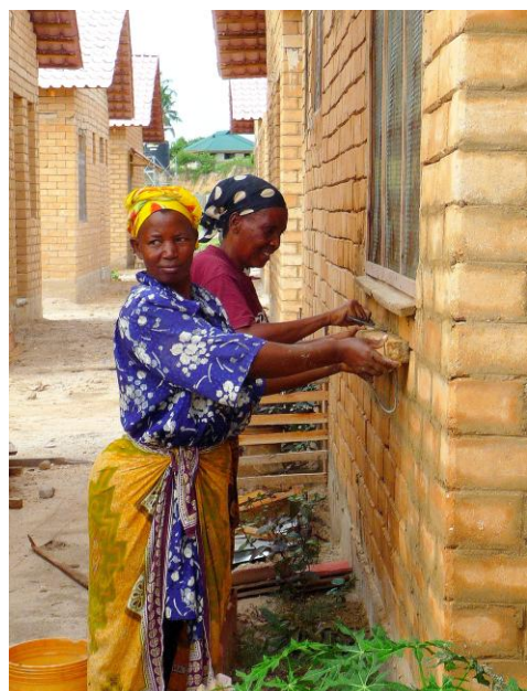
In Tanzania and Zimbabwe, around half of the builders trained during the project are women.
