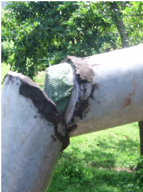
Picture 4 Broken rainwater harvesting pipe
