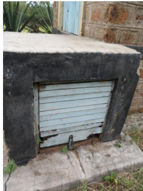
Picture 5 Wooden urine chamber door eaten by termites
