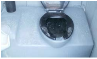
Figure 28. Holding tank in a prefabricated toilet unit.
