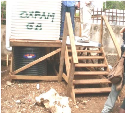
Figure 29. Single cubicle tanks
