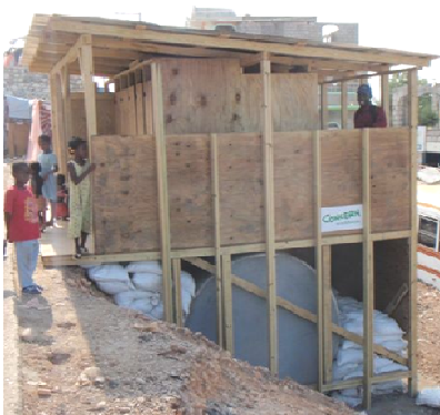
Figure 30. Multiple cubicle tanks
