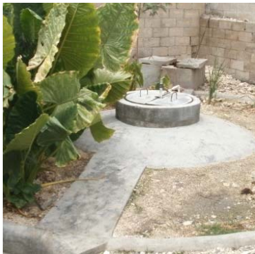
Figure 38. Biogas plant in Port au Prince
