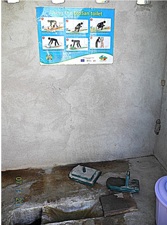
Figure 8, An UDDT squatting pan application that is molded (/casted) of concrete into the floor.
