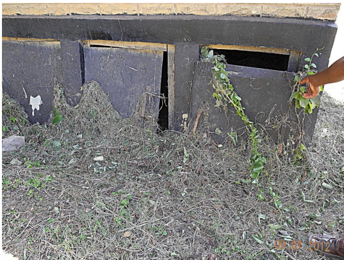
Figure 30, Vault door behind the UDDTs were disordered and some weeds were growing inside the vaults.
