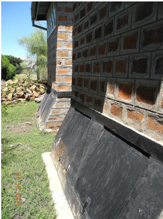
Figure 10, Back of the UDDTs: Vault doors, water harvesting system (lander and directing pipe) and ventilation holes.
