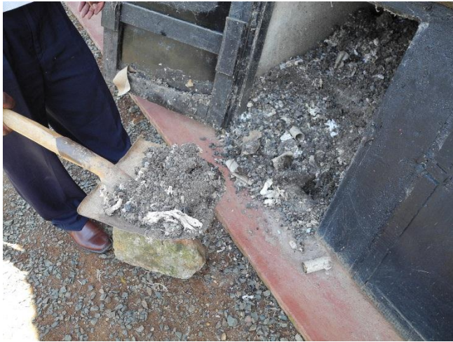
Figure 26, Faeces in the vault before the actual storing period.
