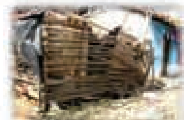
Poorly maintained individual toilet
