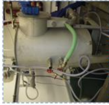
3 - Pretreatment tank Volume of tank: ~ 400 l
