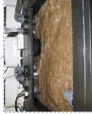
5 - Membrane bioreactor (MBR) Volume of tank 480l
