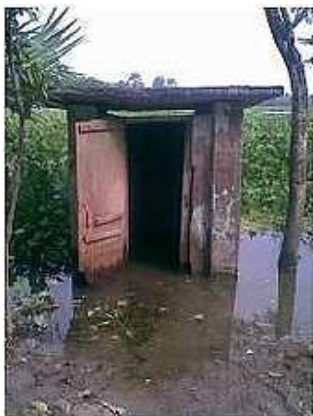
Figure 2: Unusable pit latrine during a flood in Bangladesh (source: S. Uddin, 2007) 1 .
