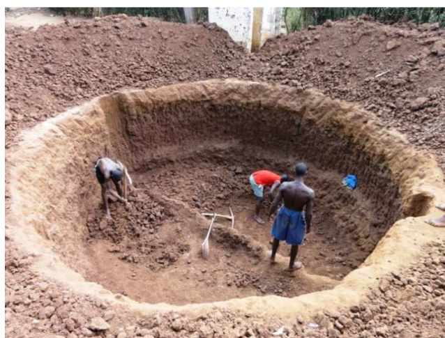
Figure 1: Excavations for a biogas digester in Livingstone, Zambia at a project of the Devolution Trust Fund (DTF) (source: P. Feiereisen, 2011)
