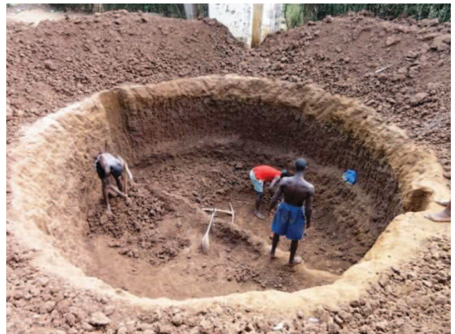
Figure 1: Excavations for a biogas digester in Livingstone, Zambia at a project of the Devolution Trust Fund (DTF) (source: P. Feiereisen, 2011)
