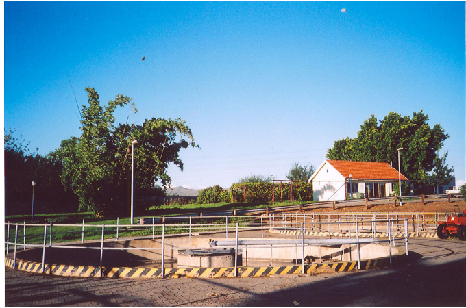
Figure 16: Gammams Wastewater Treatment Plant Source: Author's photo
