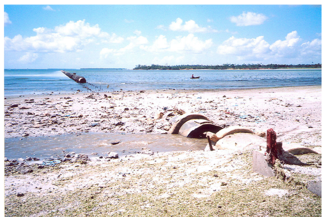
Figure 26: Sea outfall Dar es Salaam
