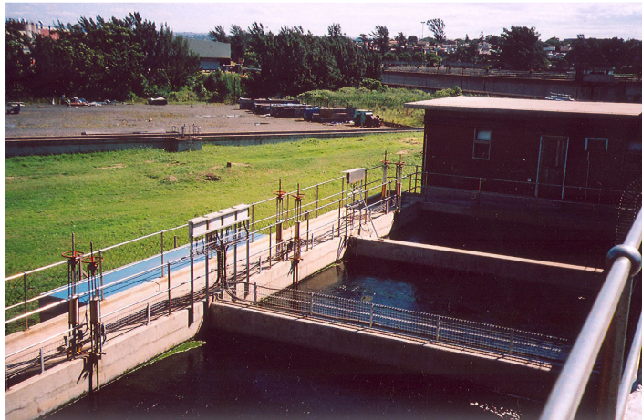
Figure 23: Veolia Wastewater Treatment Plant in Durban
