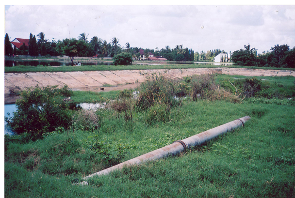
Figure 28: Silted anaerobic pond and overgrown the pond Msasani
