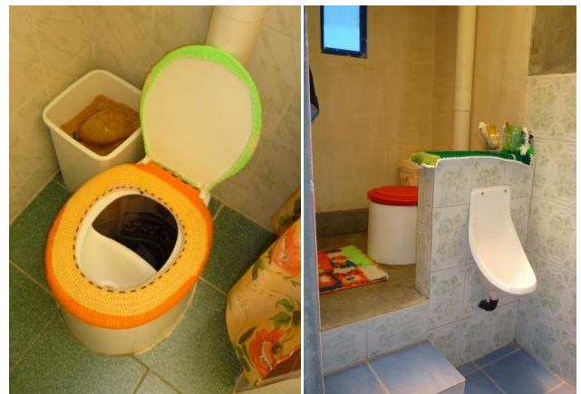
Fig. 9: View of the interior of the UDDT unit. Right picture shows also the urinal (Andersson, 2011).
