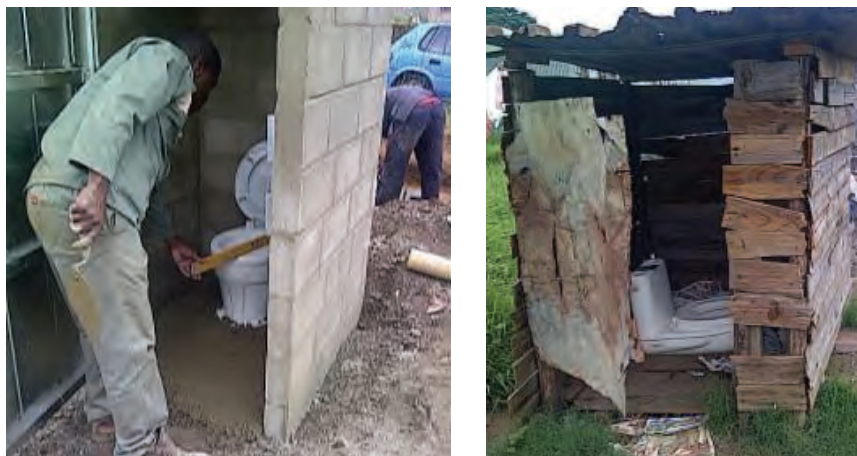
Figure 4.25 Household 11: Homebuilt latrine with HS pedestal (right). Pour flush system under construction (left).
