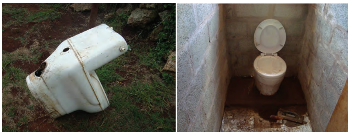
Figure 4.30 Household 16: Old HS pedestal removed (left); new pour flush system during installation (right)
