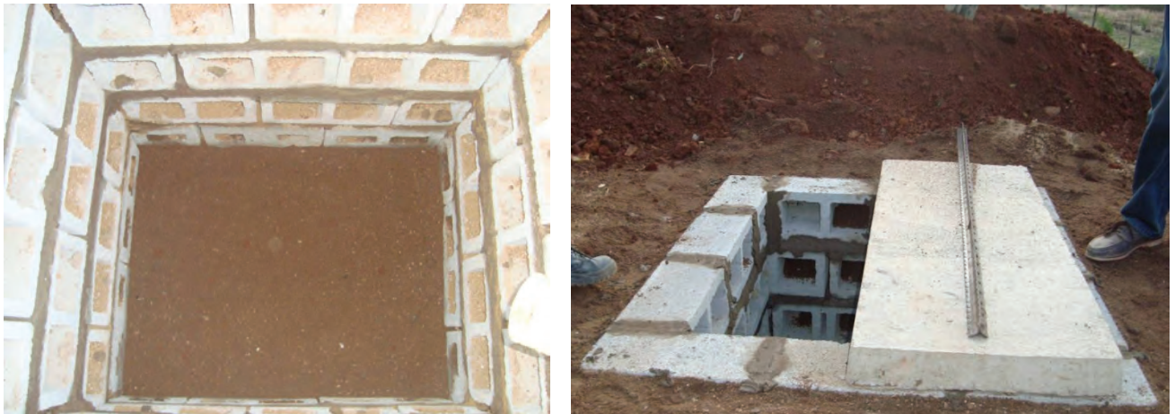
Figure 4.9 Interior of a soak pit (left). Each pit is covered by two 1.2 m by 1.4 m precast concrete slabs (right)
