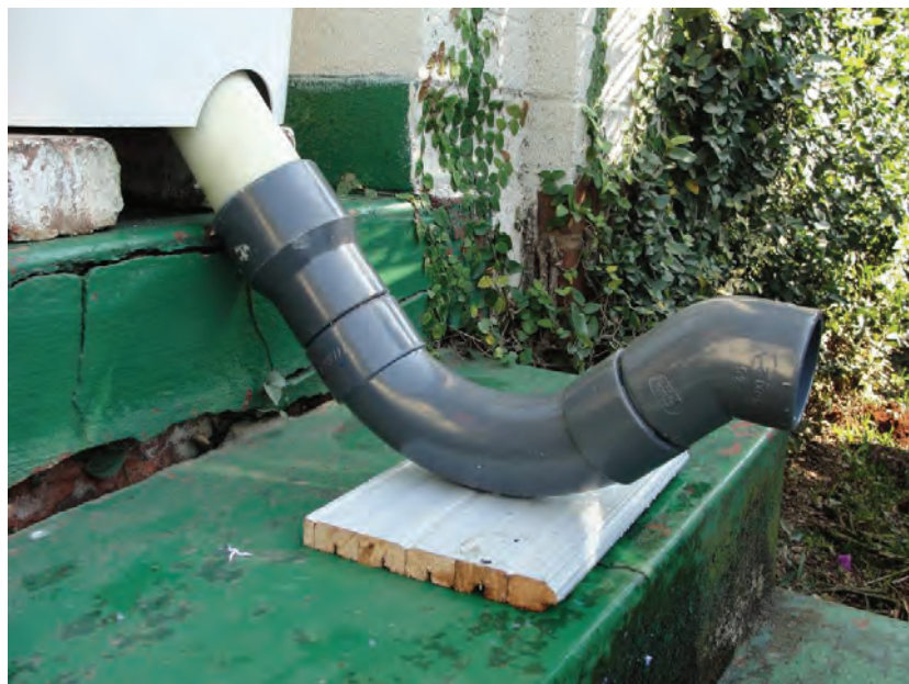
Figure 4.2 The water seal is made up using three standard 65 mm diameter PVC pipe fittings – a reducer, a long radius 90° bend, and a 45° bend
