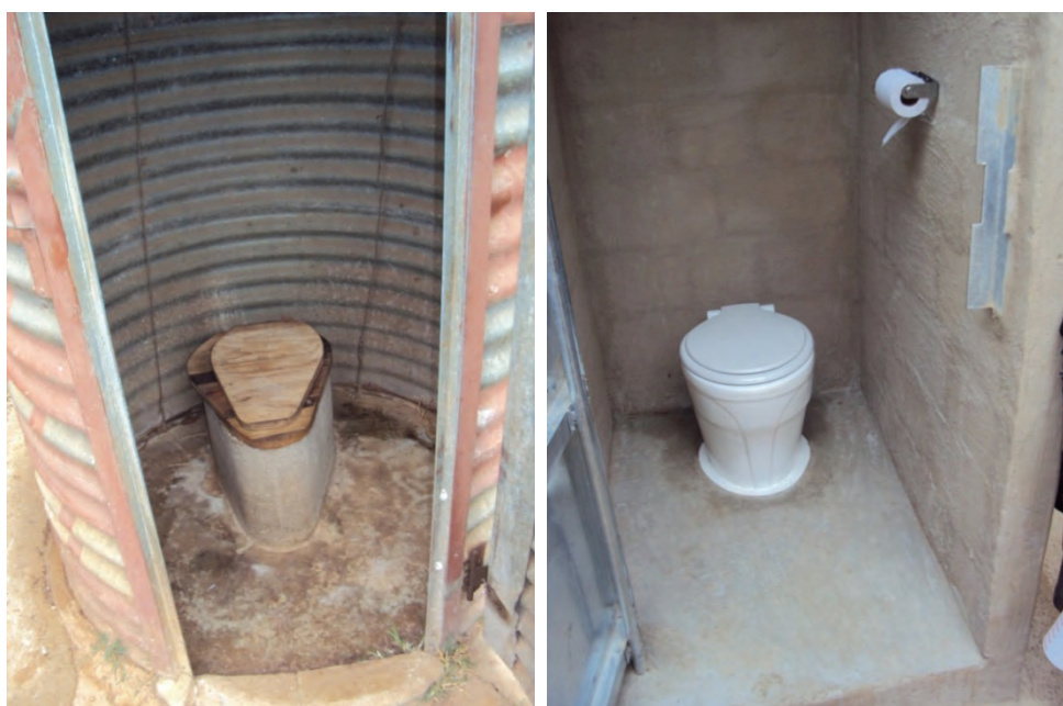
Figure 4.7 (below) Existing VIP (left) and new pour flush in structure (right) at Household 1
