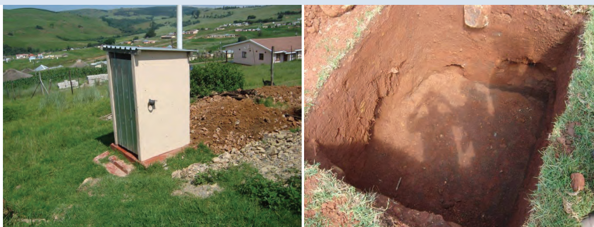
Figure 4.20 Household 6: Existing municipal VIP (left) and pour flush pit under construction (right)
