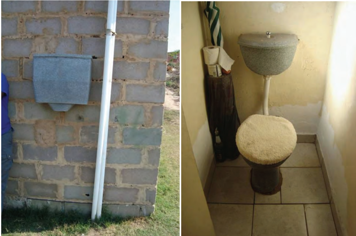
Figure 2.17 DSA reserve tank, cistern and pedestal
