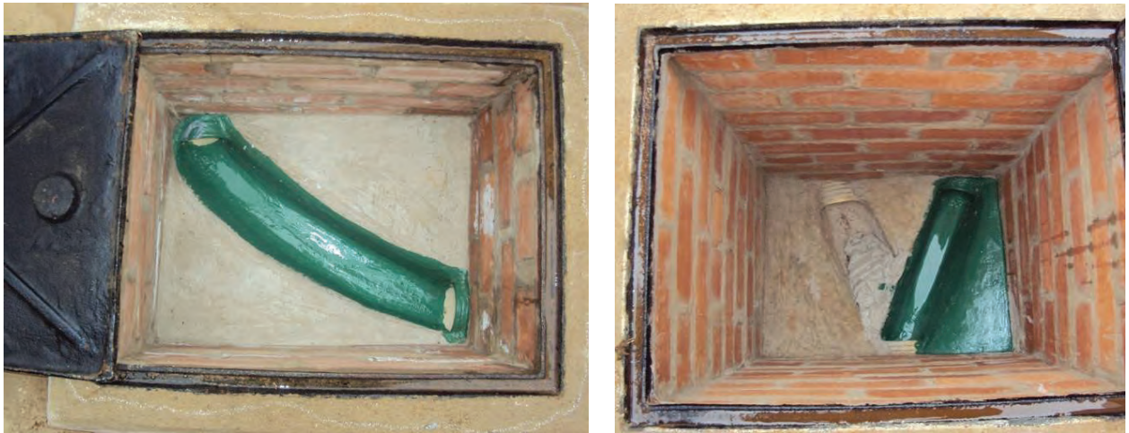
Figure 4.8 First and second junction boxes of sewer at Household 1. The second is a splitter box, where the flow is routed to either one of two leach pits using a section of PVC pipe as the switch.
