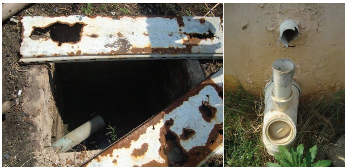
Figure 3.2 Exposed soakaway and broken pipes
