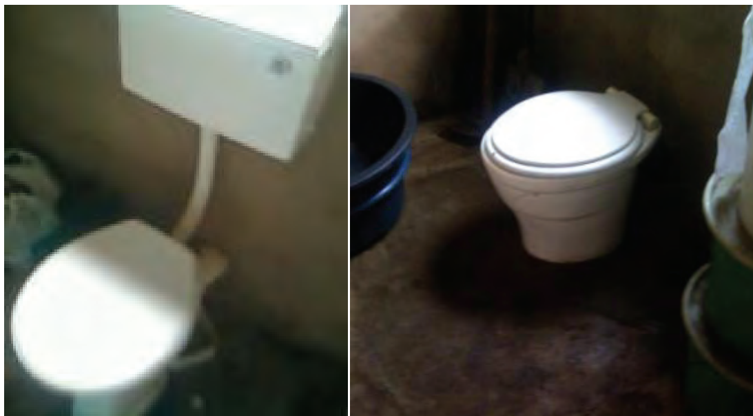
Figure 4.32 Household 18: Full flush pedestal (left) replaced with pour flush system (right)
