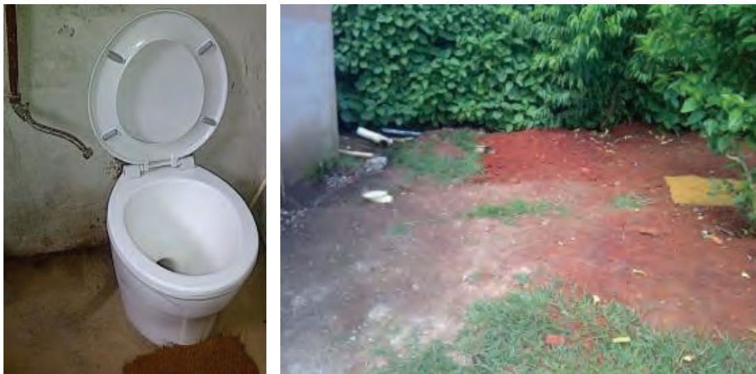
Figure 4.33 Household 19: New pour flush pedestal installed in the house (left) and soak pit constructed and covered with earth behind the house (right).
