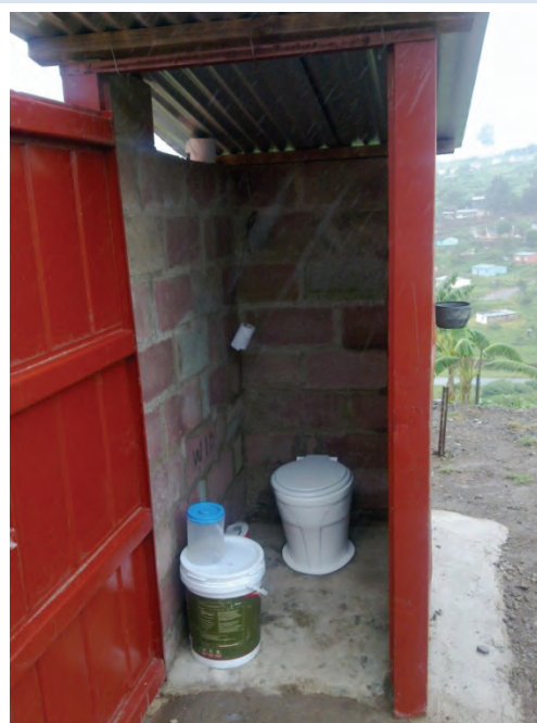
Figure 4.17 Household 3: Pour flush toilet installed in outdoor structure.
