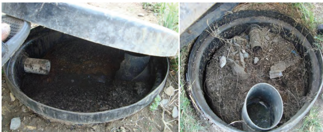
Figure 3.3 DSA liquefier tanks in Ifafa Grebe that were not properly sealed and covered with earth during installation
