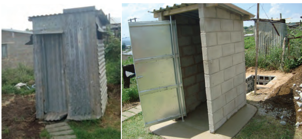
Figure 4.19 Household 5: Existing home built latrine (left) and pour flush under construction (right)
