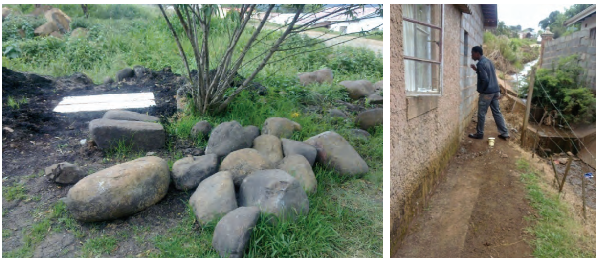
Figure 4.29 Household 15: Large rocks removed for construction of soak pit (left); soak pit installed in new extension of the house (right)
