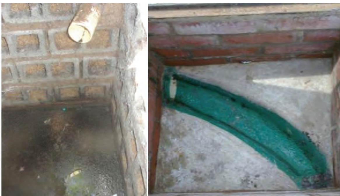
Figure 4.35 Soak pit (left) and first junction box (right) after 13 months of use
