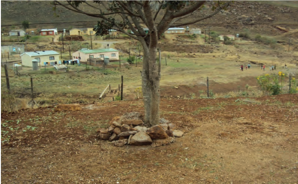
Figure 4.10 The completed soak pits (either side of the tree) are covered with topsoil. (At a later date inspection ports were added to aid with the checking of sludge depth)
