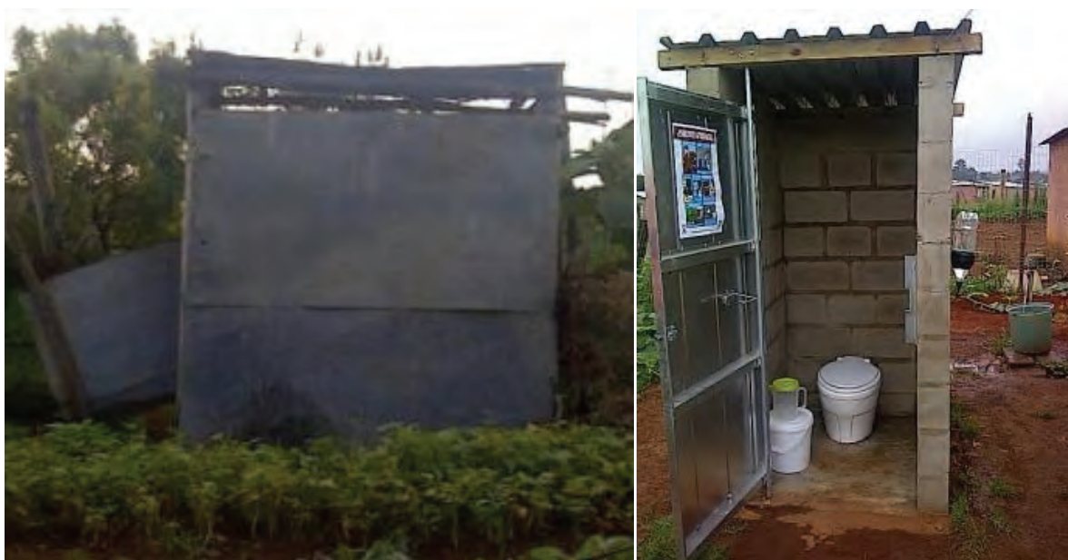
Figure 4.24 Household 10: Home built structure for a latrine at a home which was overlooked when HS systems were originally installed (left); new pour flush system (right)
