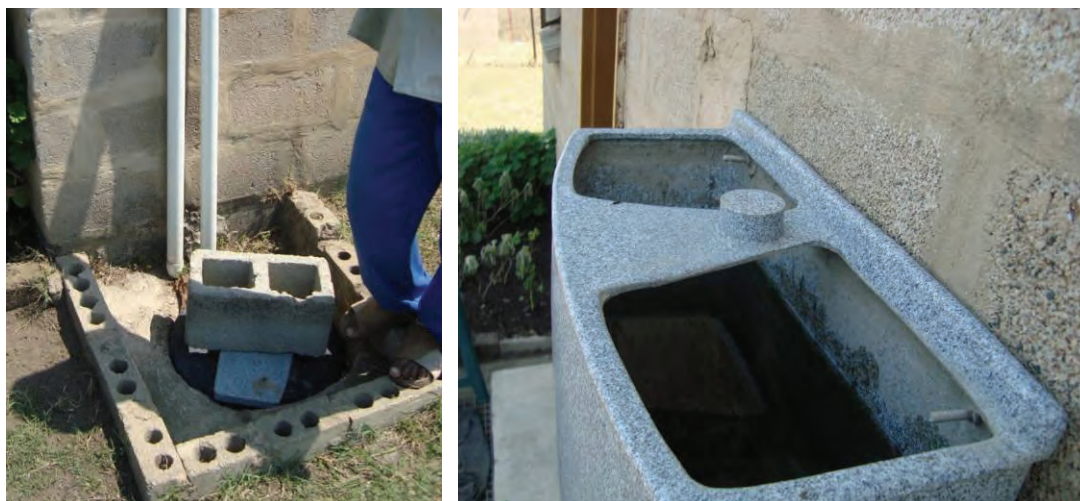
Figure 3.4 Householder has used the lid from a reserve tank (left) to seal a liquefier tank which has not been properly sealed and covered (right).
