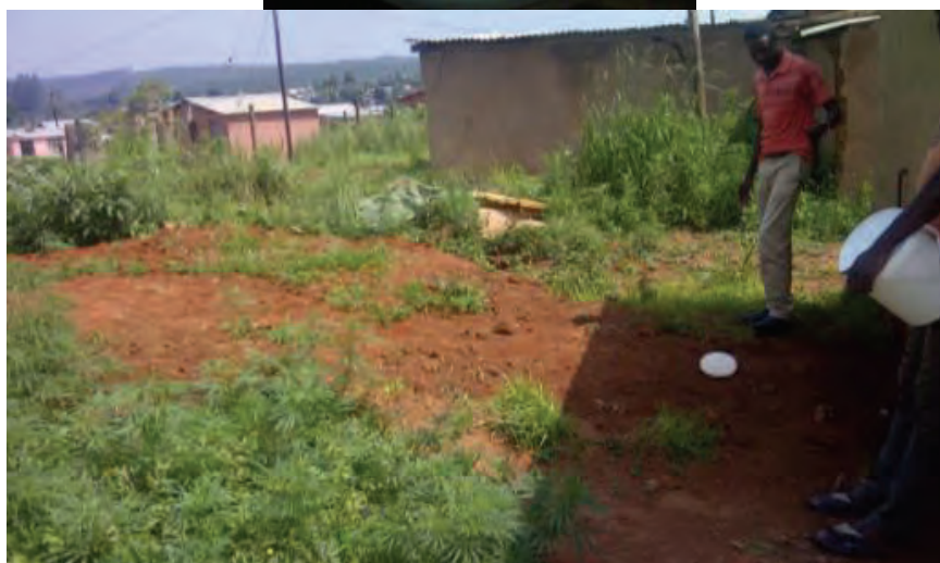
Figure 4.31 Household 17: HS system with missing tipping tray which had not been flushed because the water supply was cut off (right). Rodding eye (white) indicates sewer laid through old pit to new pit (left).
