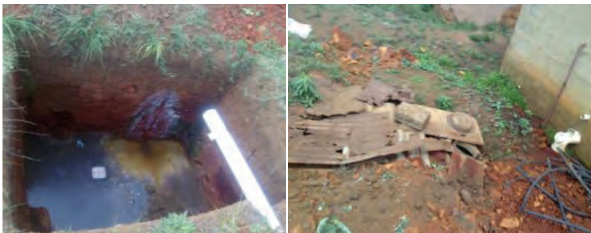
Figure 4.13 Uncovered or poorly covered soak pits in Siyathuthuka
