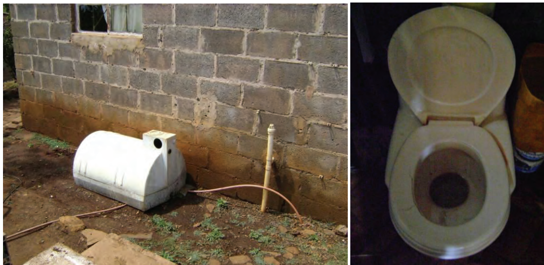
Figure 3.1 Water tank that has been removed (left) and pan with tipping tray missing (right)
