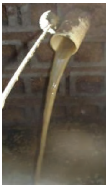
Figure 4.16 Sewer cleared after plastic packet is removed
