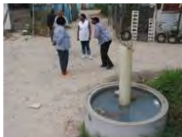
Burundi, 2005. Standpipe vandalised. Stagnant water problem
