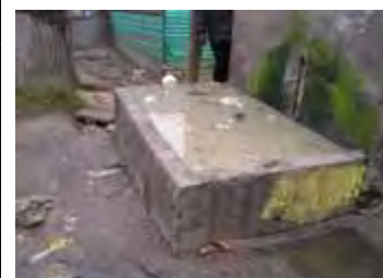
Shuku, 2005. Failure of greywater drainage rings
