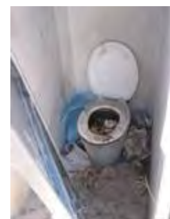
Green Park, 2005. Poor maintained toilet
