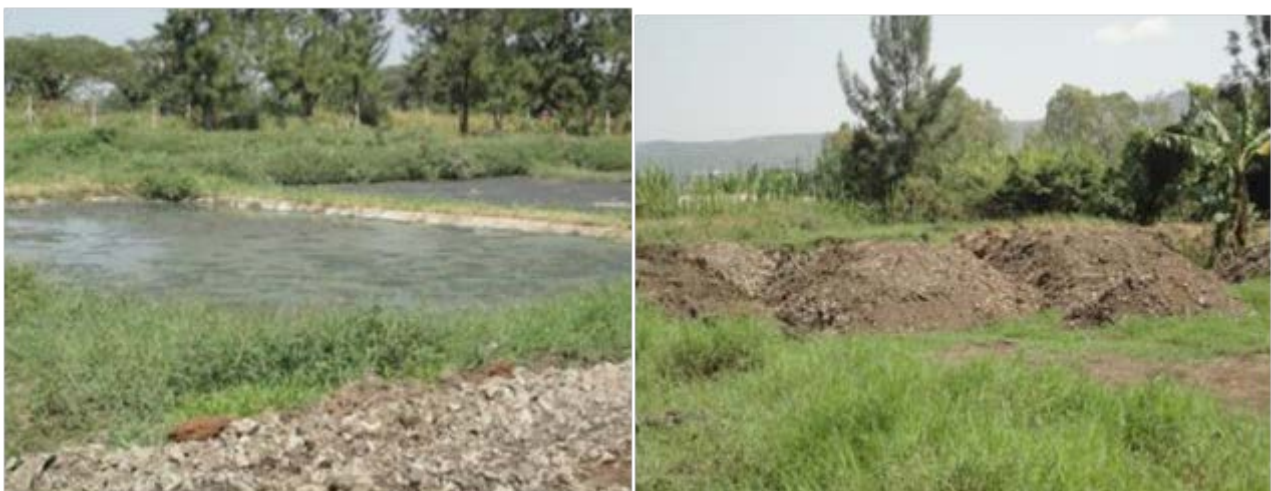
Figure 3-24 : FS Drying Beds (left) and dried FS (right) at the Kisat WWTP
