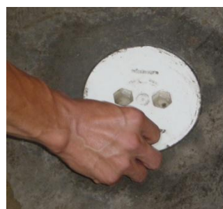
Figure 4-52. Plastic cap for access to septic tank
