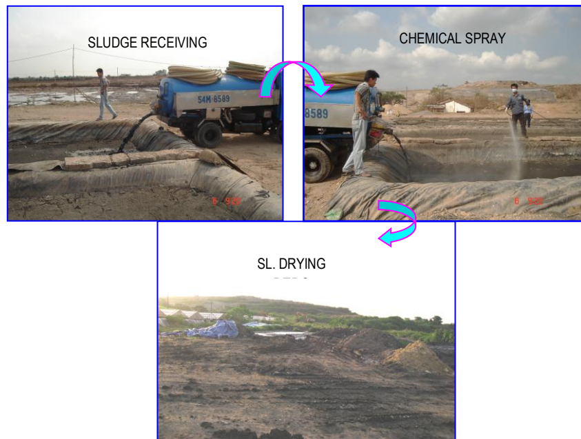
Figure 4-72. Fecal sludge treatment plant at Dong Thanh landfill
