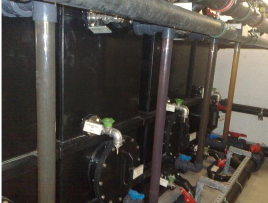
Figure 11 Urine storage tanks
