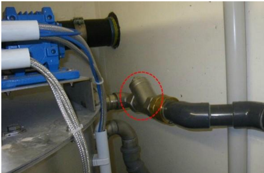
Figure 14 Dirt trap of the MAP reactor (Source: GIZ, 2011)
