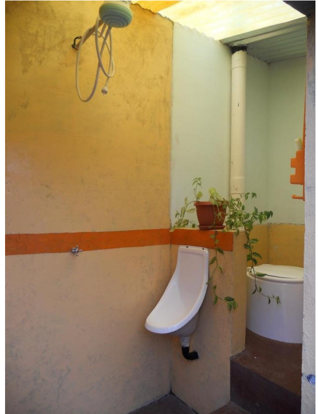
P.2 The interior of a one door Ecological toilet in District 7. 9
