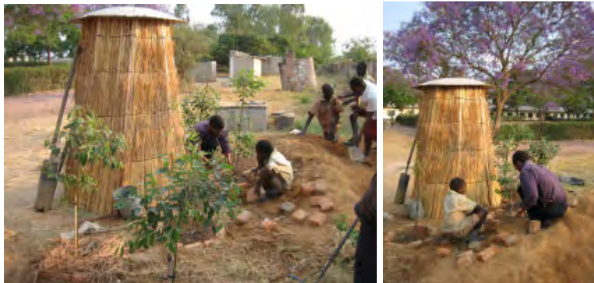
Two toilet pits were encircled by gum trees at the school in October 2009.
