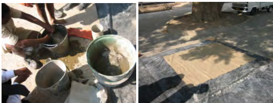
The cement paint is prepared and the hessian sheet laid on plastic sheet,
