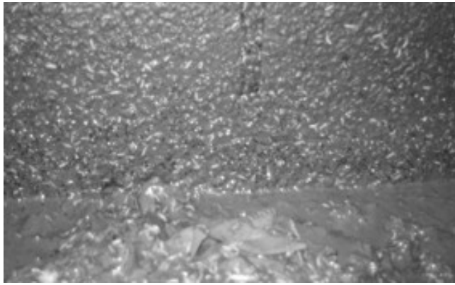
Walls of pit during emptying. This pit contained a very high load of maggots due to the fact that the ventpipe was missing.
