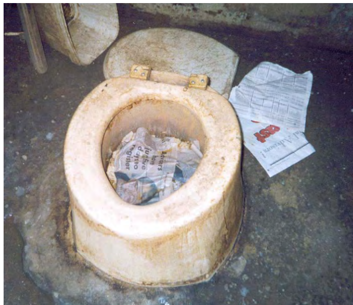
Figure 1.1: Photograph of a poorly maintained, overflowing pit latrine, filled with non-biodegradable material.
