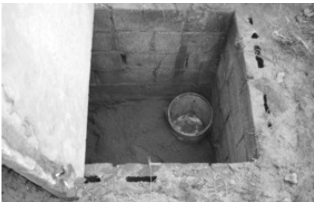
A pit latrine after emptying has been completed. This pit latrine was fully lined with open vertical joints in the block work
