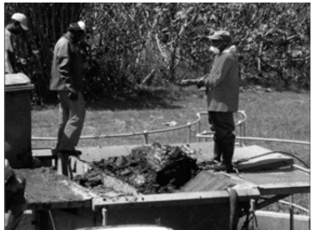
Converted skip with grids for separating solid waste from faecal sludge. Separation is achieved with the assistance of high pressure water spraying
