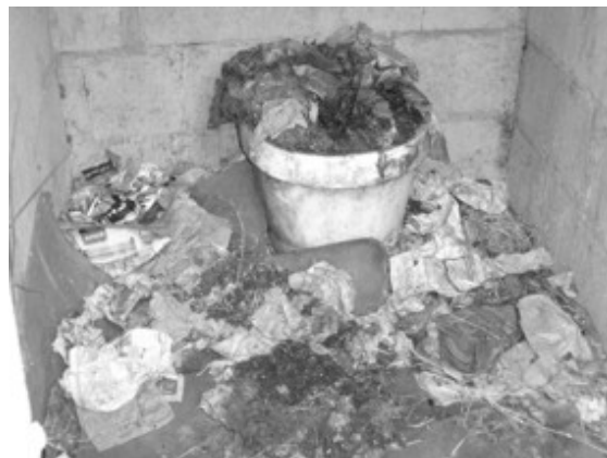
Overflowing pit latrine: the superstructure has become an extension of the pit.
