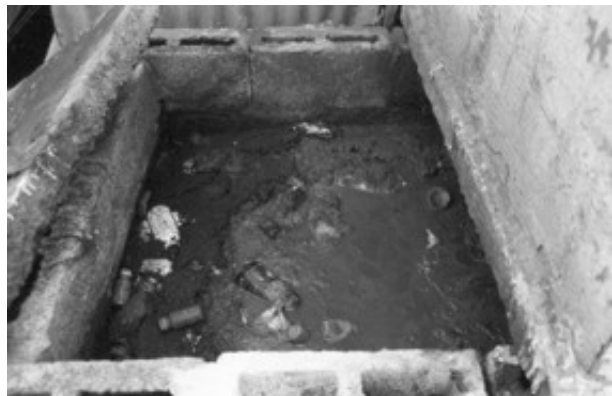
Corresponding pit contents of overflowing VIP latrine viewed through the opened back plate
