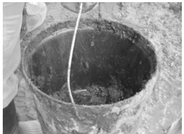
Pit contents are transported to 200 l wheel bins
