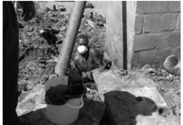
Worker inside pit latrine with minimal protection
