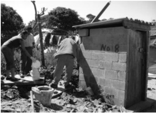
Project team standing by to take samples from different depths within the pit
