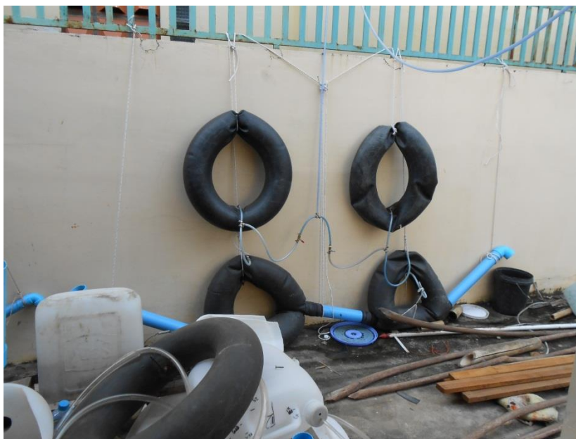
Figure 20. The two tyres at the lowest position on the wall connected with blue pipes are the digester. The two tyres above function as gas reservoirs.
