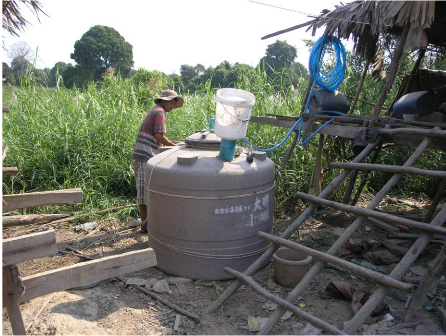
Figure 19. Hard plastic dome biodigester.
