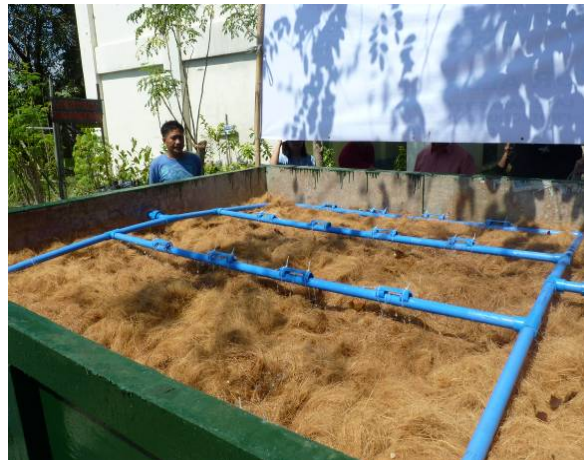
Figure 2. Cocopeat biofilter with distribution pipes (blue) constructed for Putatan Elementary School
