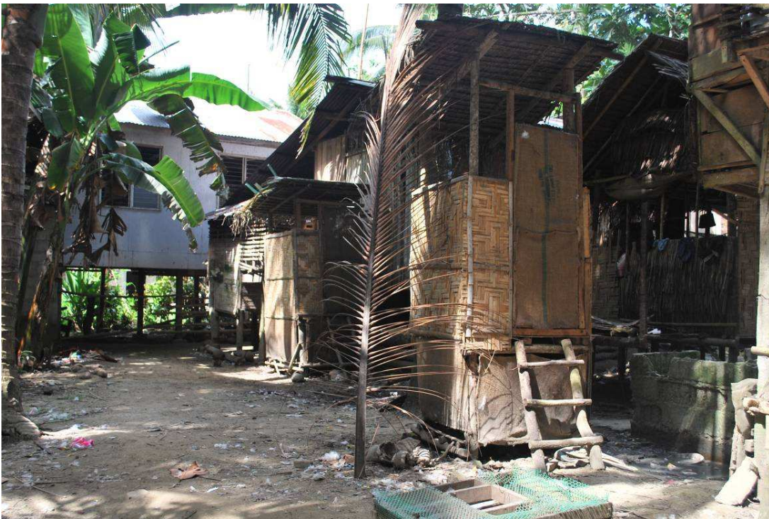
Photo 3. View of a detached single-vault ecosan toilet.
