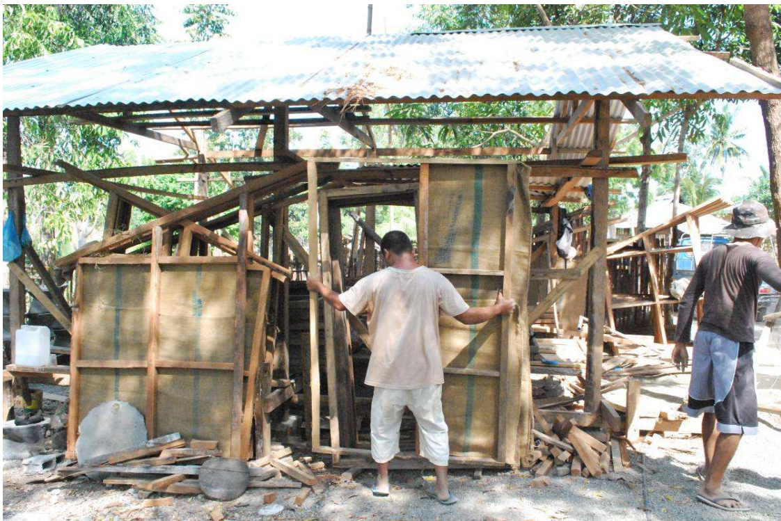
Photo 4. Pre-fabricating walls of ecosan toilets is our production area in Libertad Municipality.
