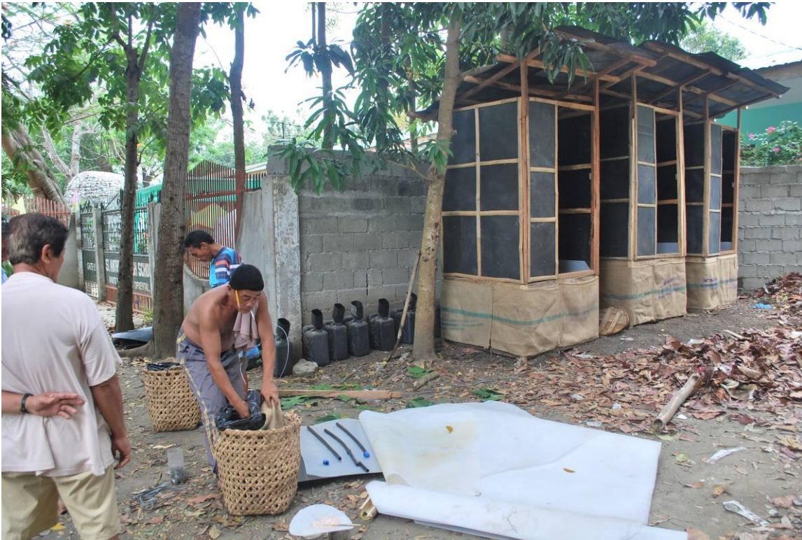
Photo 26: Installing the pre-fabricated units. Rattan basket is used for feces collection. Eco-Pees or male urinals lined at the side of the concrete fence.
