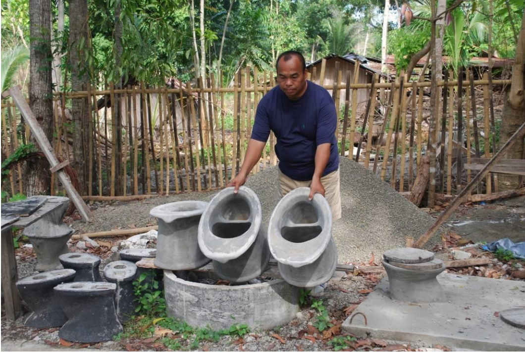
Photo 4: Our ecosan bowl is made of cement, sand and gravel reinforced with wire. The mold used to form the toilet bowl is also made of cement. One bag of cement can produce 6 of these bowls.
