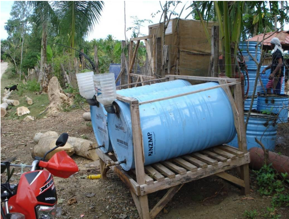
Photo 19: Recycled drums are used for urine, rainwater and grey-water collection. Recycled drums can be plastic or steel. In our case we are using steel which is cheaper than plastic although the advantage of the plastic is that it does not rust.
