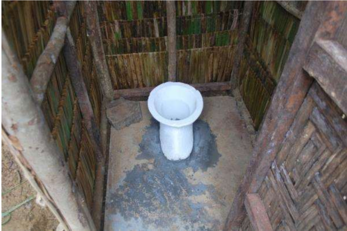
Photo 13. Inside the arborloo. Spartan and functional. Total cost is 45 USD.
