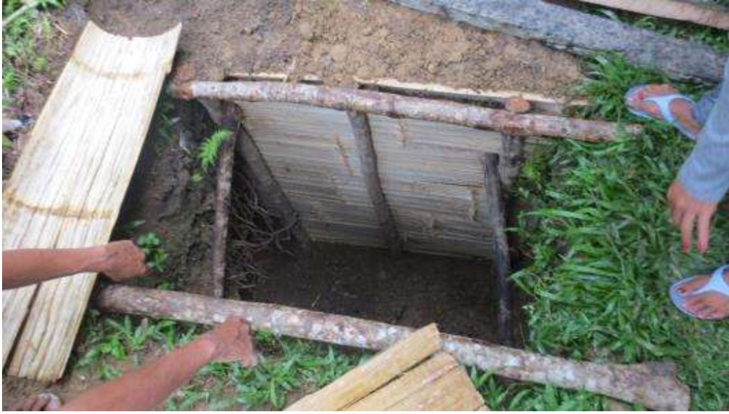
Photo 11. If soil is loose, the pit is lined with bamboo matting to support the sides.
