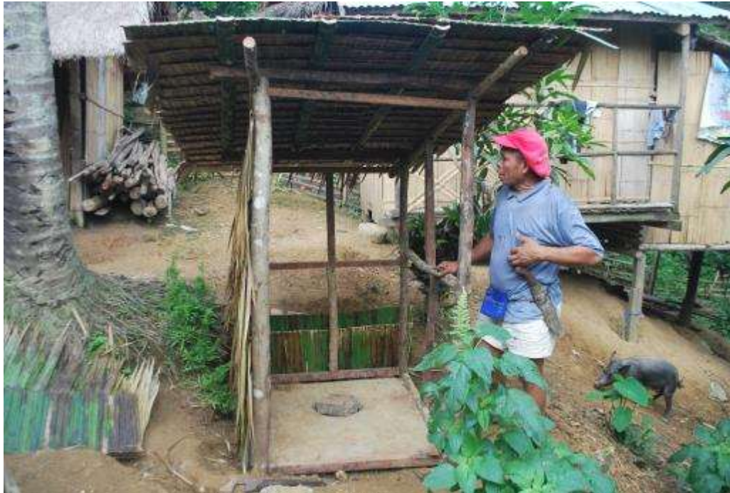
Photo 15. The superstructure is made entirely of wood poles coming from the vicinity.
