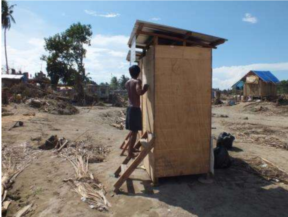
Photo 2. Single-vault ecosan toilet in a typhoon-devastated area.
