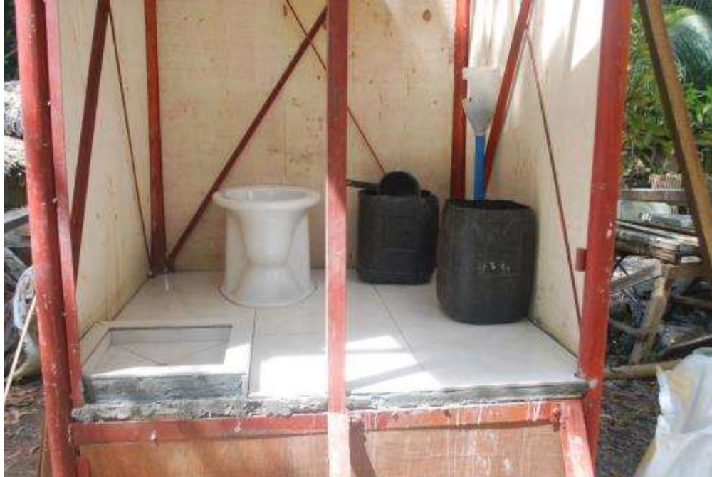
Photo 7. Inside the stee-framed single-vault ecosan toilet.
