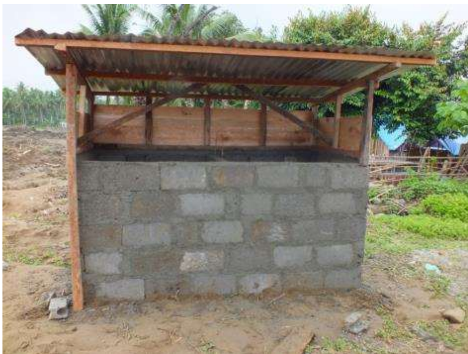
Photo 19. Cement storage boxes.
