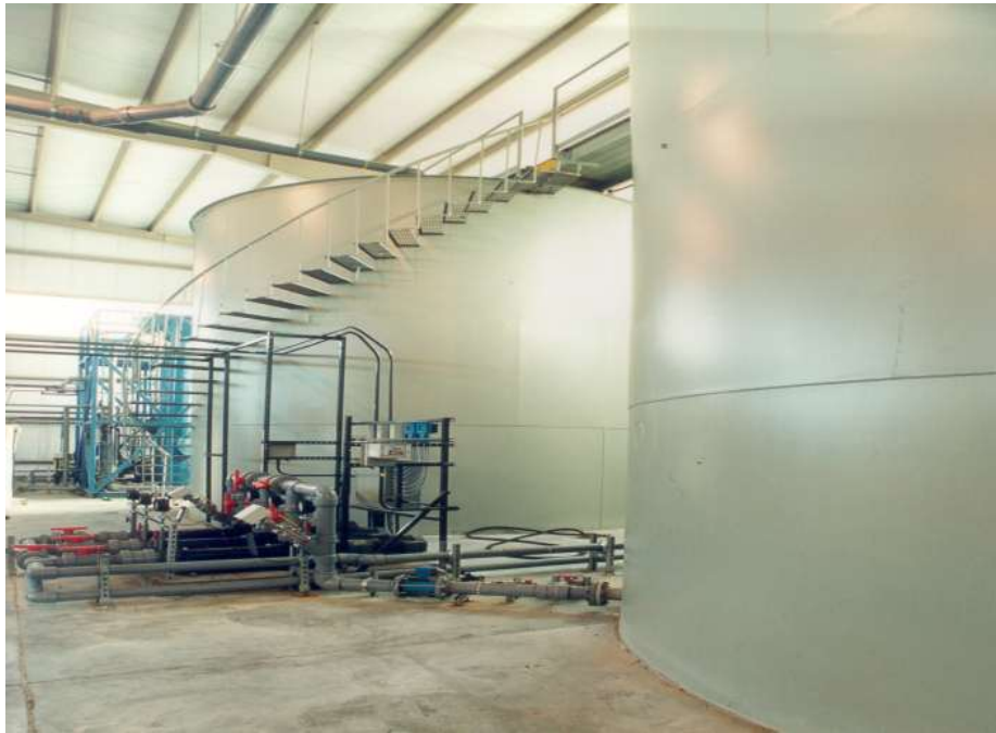
PDS fermentation and storage at 26 th Ward WPCP in New York City, 2002
