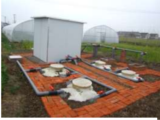
Figure 7 the onsite blackwater reuse system
