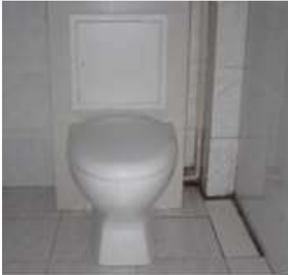
Figure 4 vacuum toilet installed in villager families.
