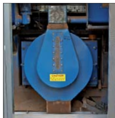
wood pelleting unit
