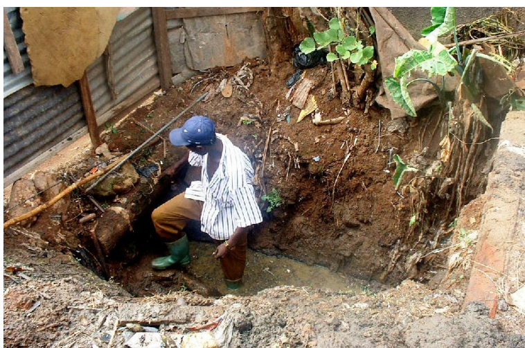
A worker fixes a septic tank in an informal settlement of Kampala City, Uganda. Photograph © Hydroconseil
