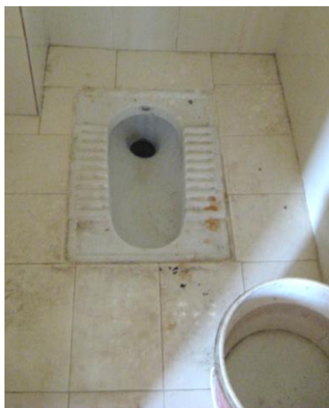
Fig. 8: Pour-flush toilet within a newly constructed community toilet (source: Keller 2009)
